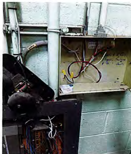
Photo 4: Current state of communication wiring
