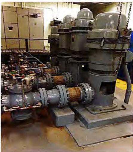
Photo 2: Gander Lakeside aged pumps
