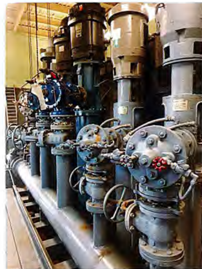
Photo 5: Gander Reservoir Pumphouse aged pumps
